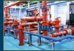
Fire Fighting System
